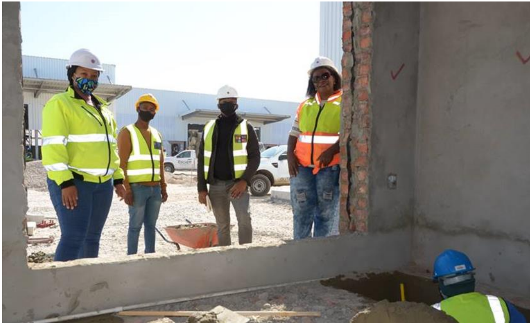
Nomdi's Construction, an SMME working at the Coega Special Economic Zone, multi-user facility Phase 2, Zone 3.
