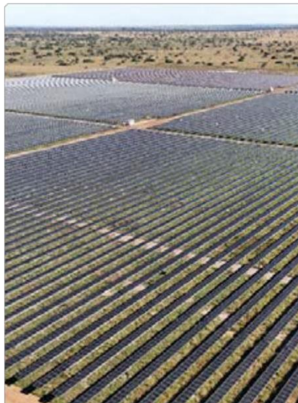
Solar panel farm.
